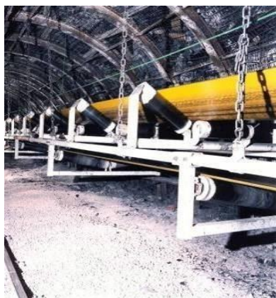
Conveyor correctly suspended and aligned.
