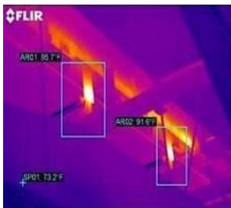
Belt edge temperature raised due to rubbing structure.
